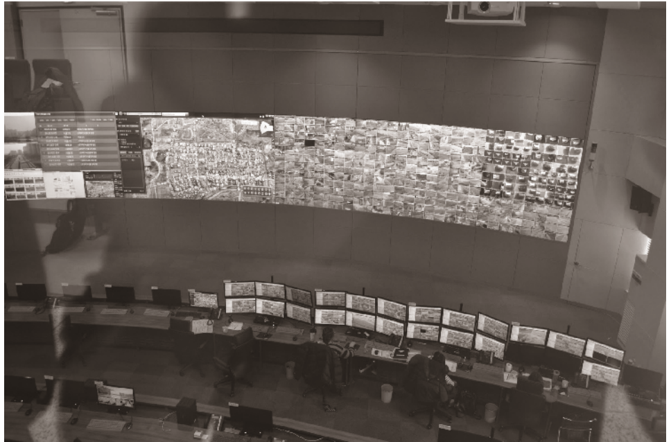
New Songdo Smart City Control Center
